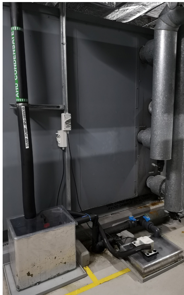
▲ Fig. 7. Photo of AHU condensate collection system
