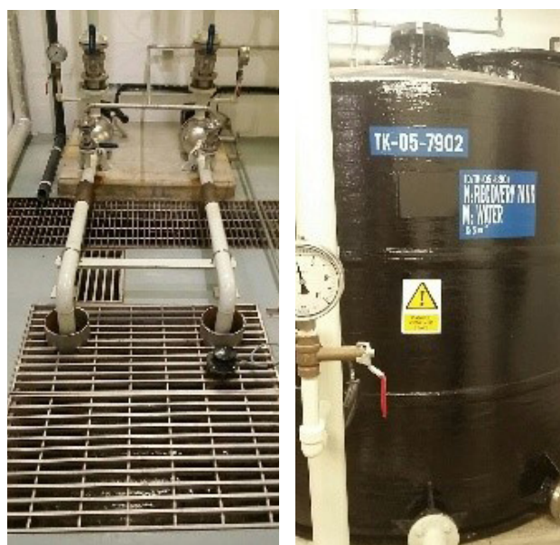
▲ Fig 9. Sump pit and recovery tank used to store reject streams from UF and RO before reuse
