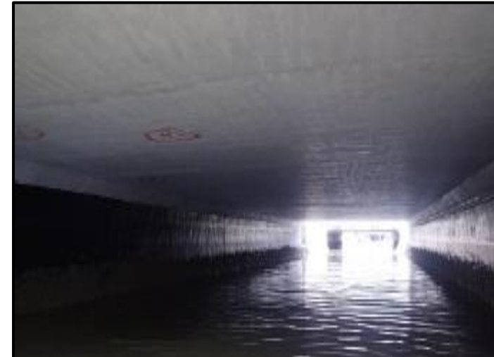
Partially Submerged drains
