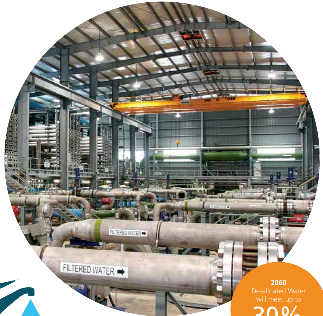
SingSpring Desalination Plant
