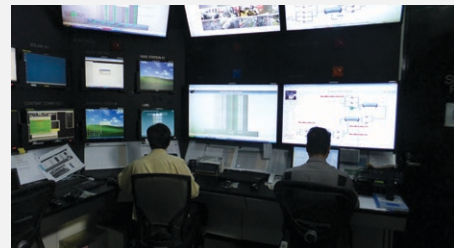
An integrated fault and building management system
