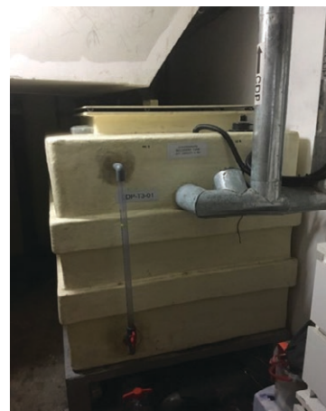
Condensate collection tanks for Hotel Towers 1 & 2 (top) and Hotel Tower 3 (bottom) at Marina Bay Sands Pte. Ltd.
