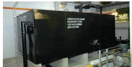
An example of AHU condensate reuse at Khoo Teck Puat Hospital
