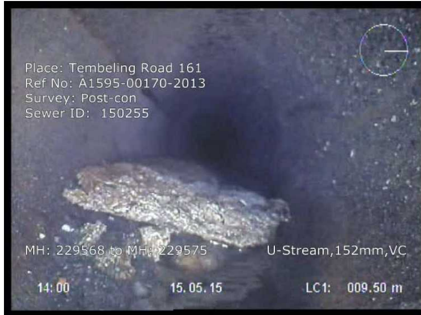
Photo: 150255-051515-S4.JPG, 00:03:31 9.5m, Debris, Stone, 20% cross-sectional area loss
