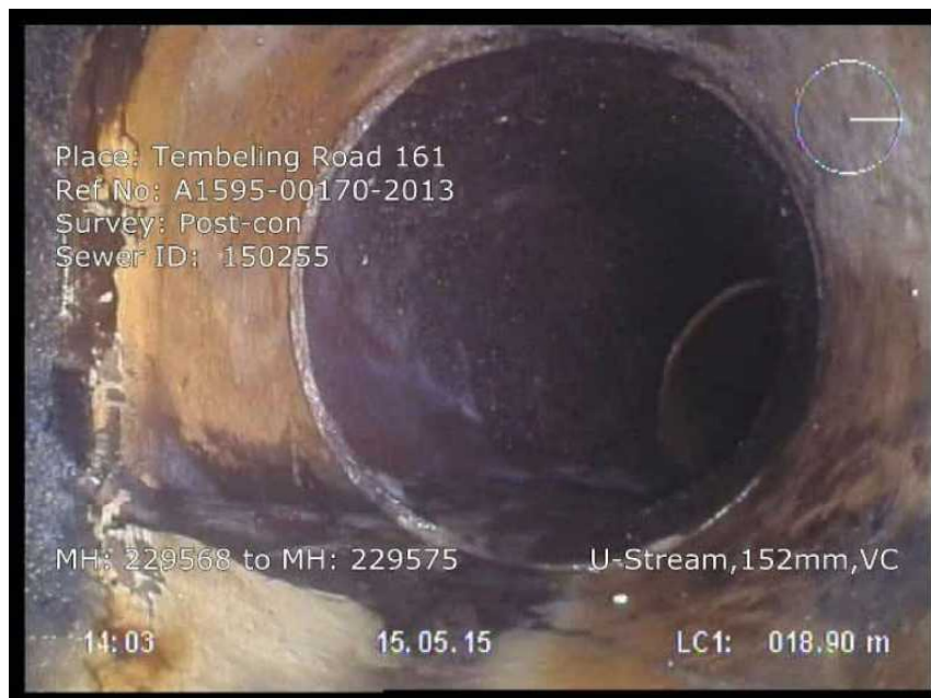
Photo: 150255-051515-S6.JPG, 00:06:01 18.9m, Connection, at 2 o'clock, 150mm diameter
