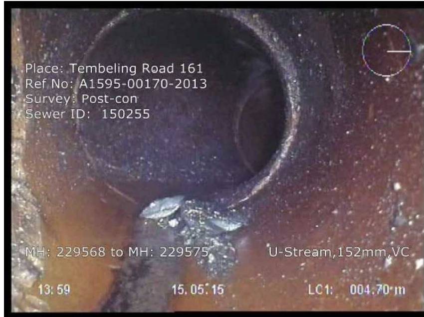
Photo: 150255-051515-S2.JPG, 00:01:50 4.7m, Connection, at 2 o'clock, 150mm diameter
