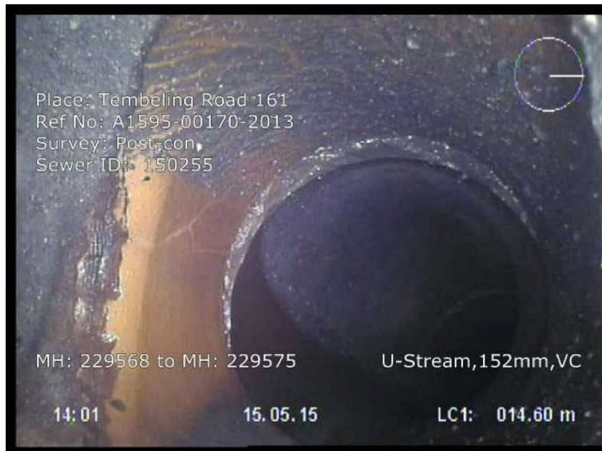
Photo: 150255-051515-S5.JPG, 00:04:46 14.6m, Connection, at 2 o'clock, 150mm diameter
