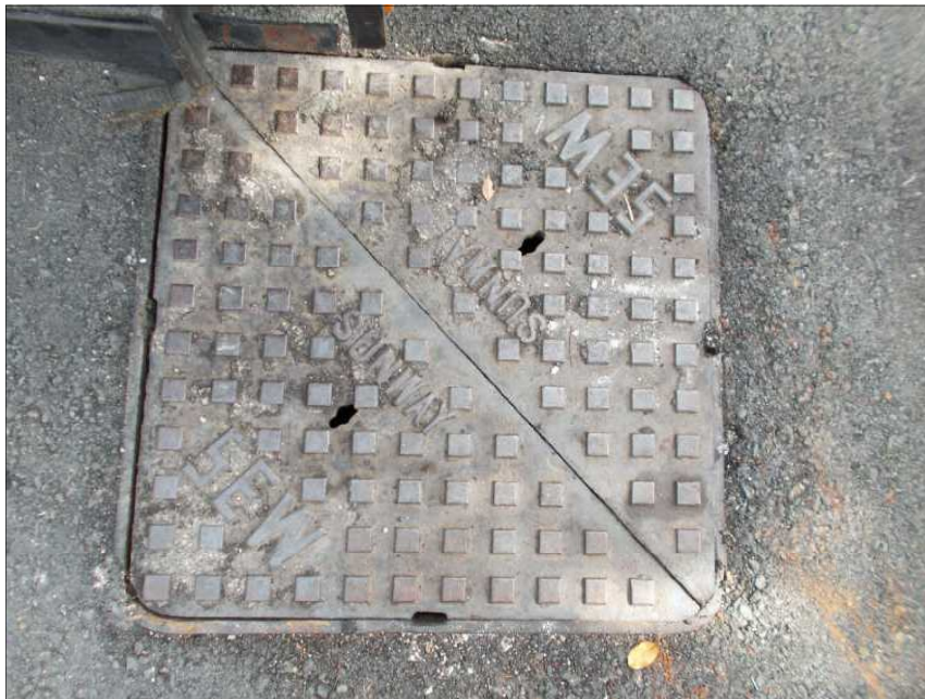
Photo: 244988-042415-M1.JPG General photograph, manhole cover
