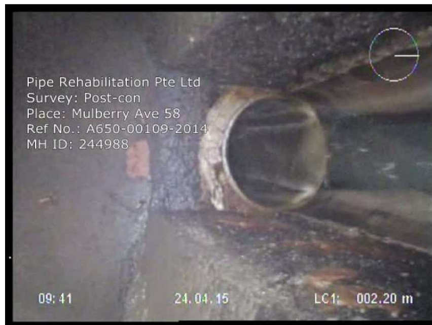
Photo: 244988-042415-M9.JPG General photograph, outgoing pipe
