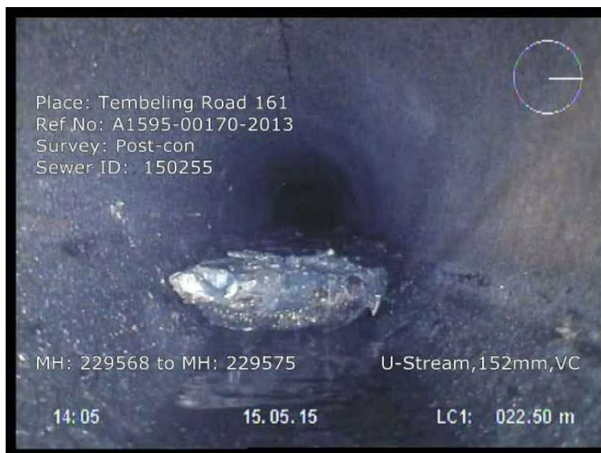
Photo: 150255-051515-S7.JPG, 00:08:17 22.5m, Debris, Cement, 20% cross-sectional area loss
