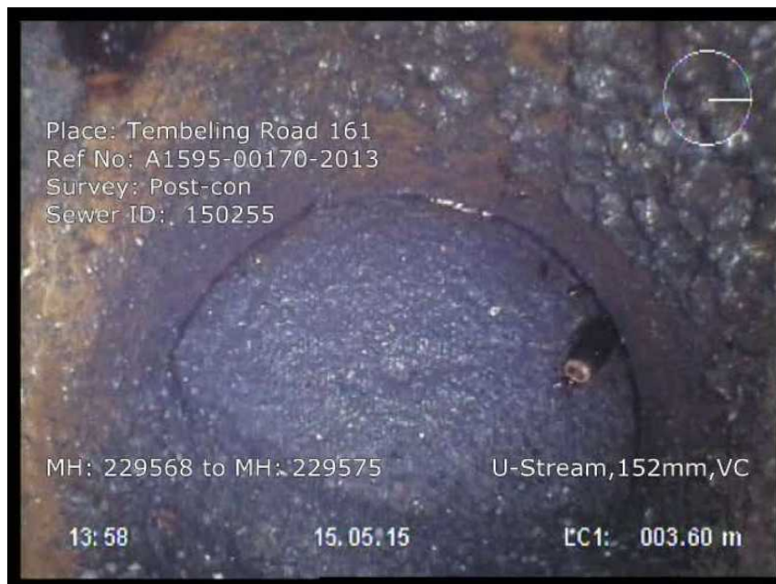
Photo: 150255-051515-S1.JPG, 00:01:25 3.6m, Connection, at 2 o'clock, 150mm diameter
