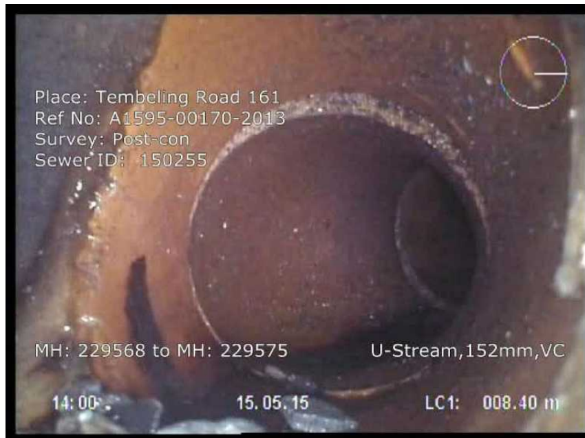
Photo: 150255-051515-S3.JPG, 00:03:06 8.4m, Connection, at 2 o'clock, 150mm diameter
