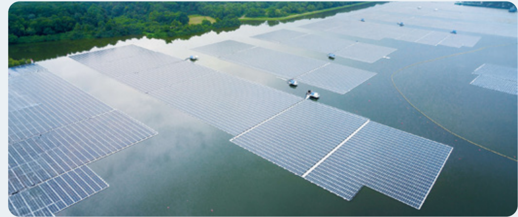
Tengoh Floating Solar Farm (photo credit: Sembcorp Industries).
