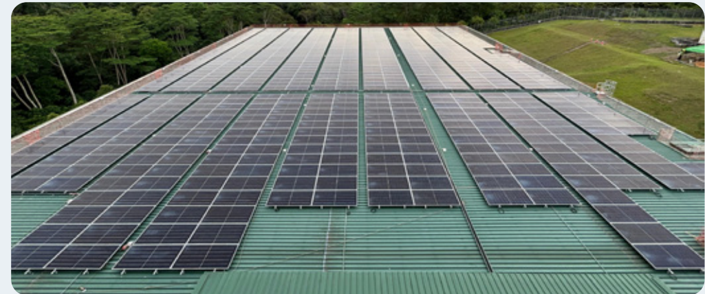
Rooftop solar panels on PUB's premises.
