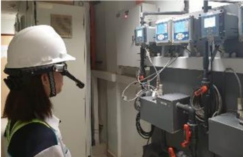
Fig 2. Hands-free smart headsets for maintenance workers allows for remote supervision by operators in real-time
