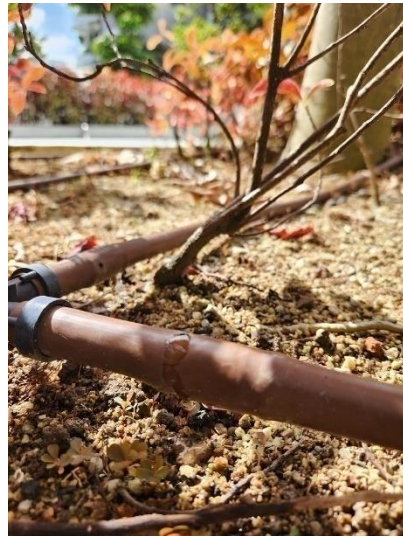
Caption: Reject water from the RO systems used to prepare dialysis water is recovered and used for irrigation.
