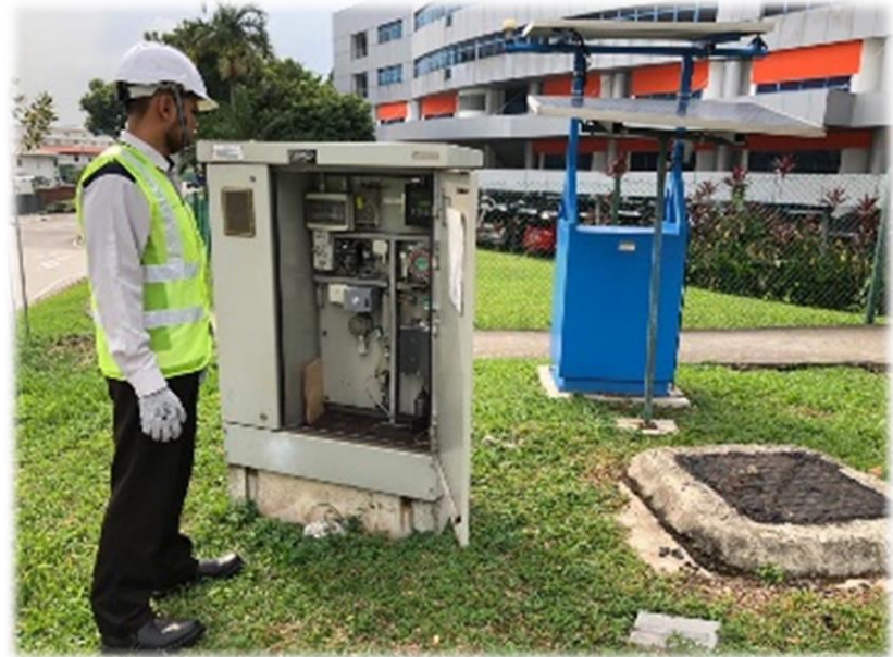
PID sensors deployed above ground
