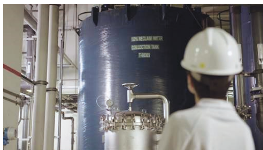
Figure 7 and 8 from top to bottom: (i) View of UMC (Singapore branch) headquarters and (ii) Reclaim Water Collection Tank
