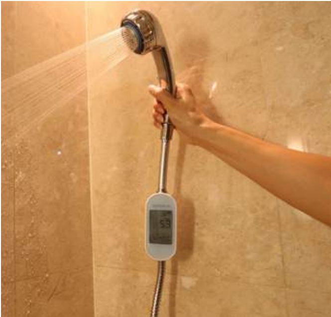
Fig. 1: A smart meter is installed on the showerhead to track water usage
