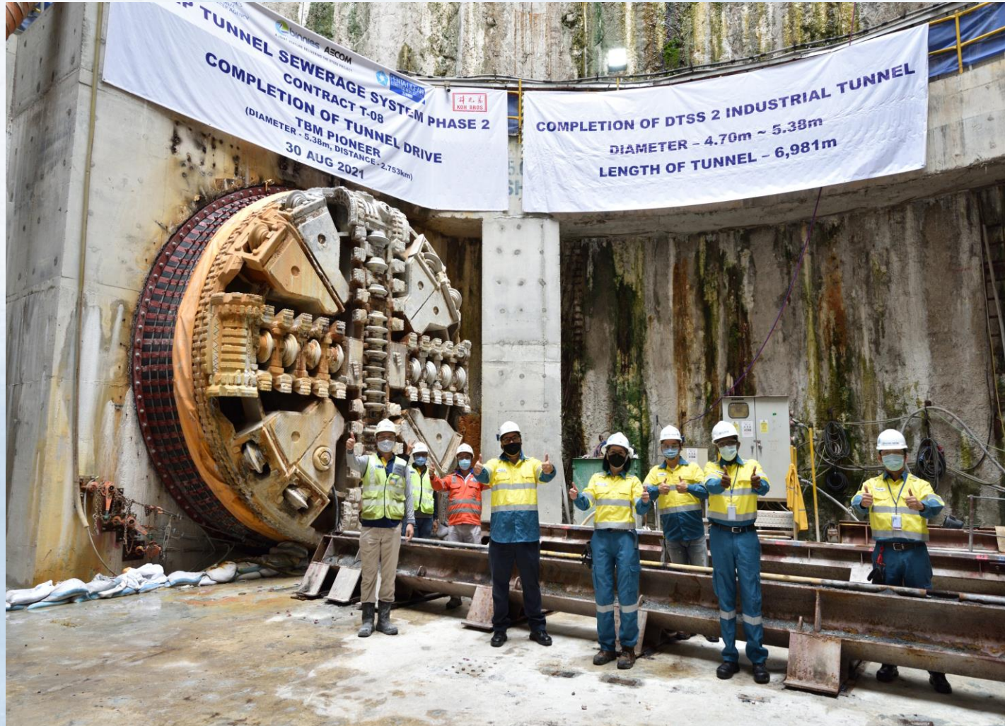
Marking the completion of the Industrial Tunnel with breakthrough of TBM Pioneer at Shaft V3 (Pioneer Road) Front Row, Left to Right: Project Director Toshio Araki (POKB JV), Director Yong Wei Hin (PUB), Chief Engineer Woo Lai Lynn (PUB), Project Director Dr Ganeshan (Binnies + AECOM JV), Deputy Project Director Benson Tan (Binnies + AECOM JV).
